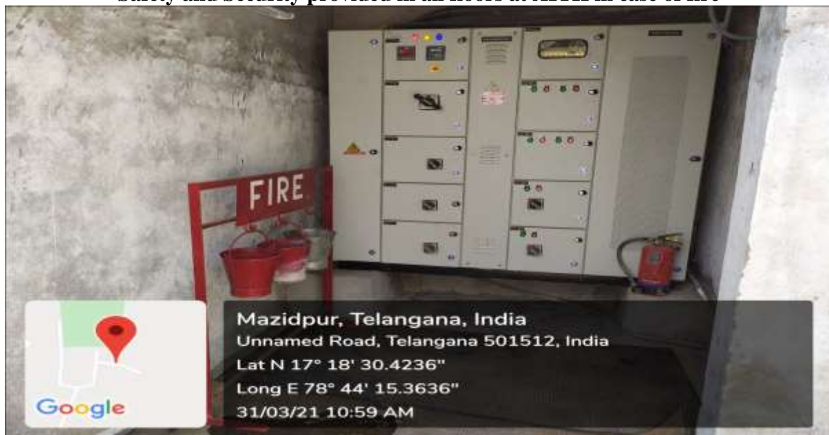
Fire safety provided at AITH
