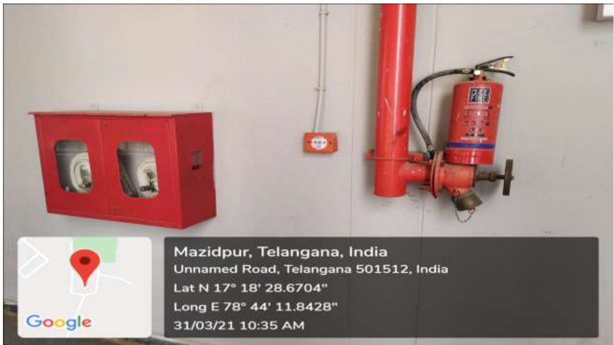
Safety and Security provided in all floors at AITH in case of fire
